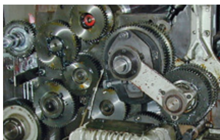
The old mechanic coupling has a complicated and irregular slip adjustment system and the drive gears are subject to wear.
